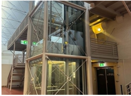
Lift in the Main Hall
